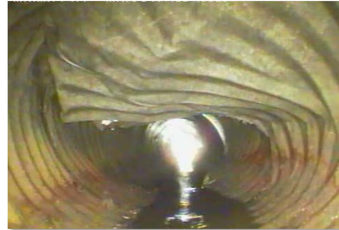
Renewal of storm sewers is a major focus of the Business Plan
