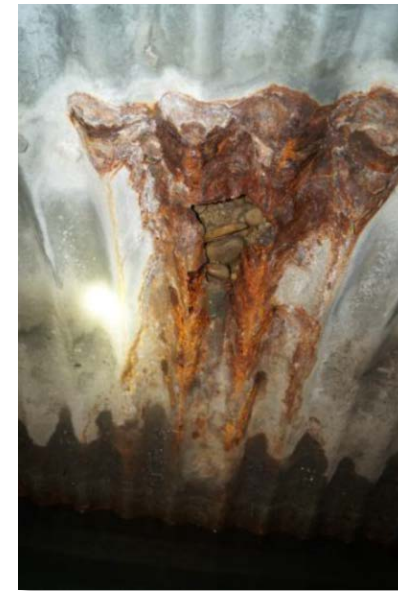
Corroded metal storm sewers require replacement
