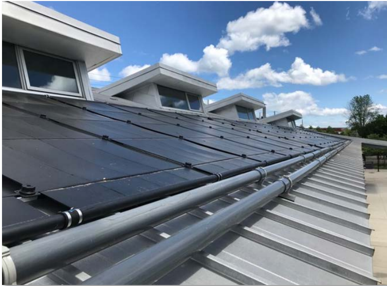
Lions Club Outdoor Pool – Solar Water Heating System
