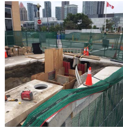
City Centre Transit Terminal, Rathburn Rd – LRT Early Works- Alectra, PSN, Rogers Joint Use Trench (JUT)
