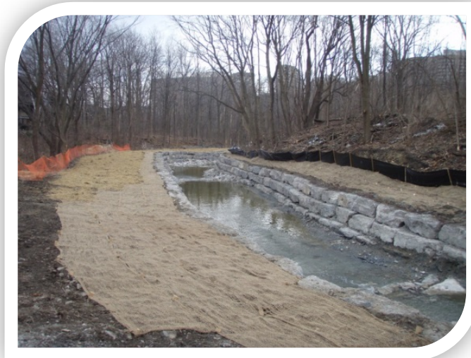
Cooksville Creek erosion control project from Burnhamthorpe Road to Mississauga Valley Boulevard
