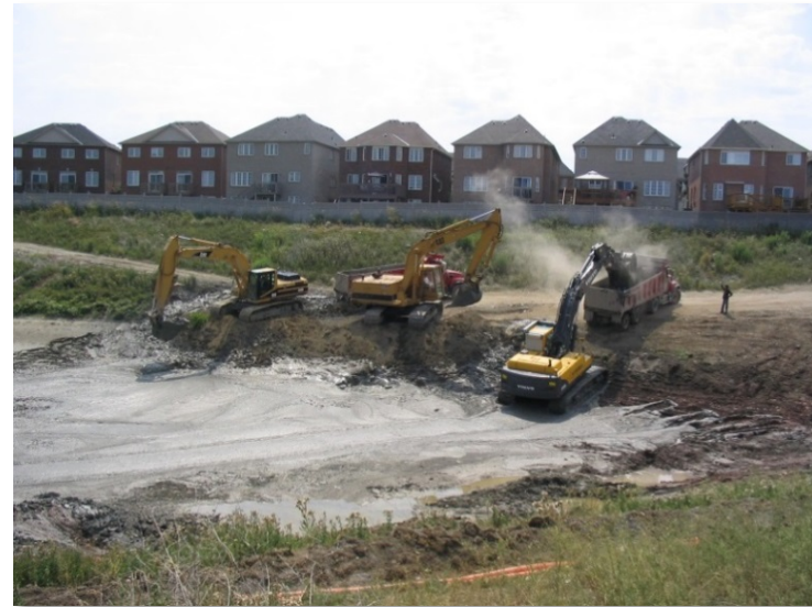
Stormwater Management Facility #5803 located southwest of Winston Churchill Boulevard and Artesian Drive is dredged of sediment
