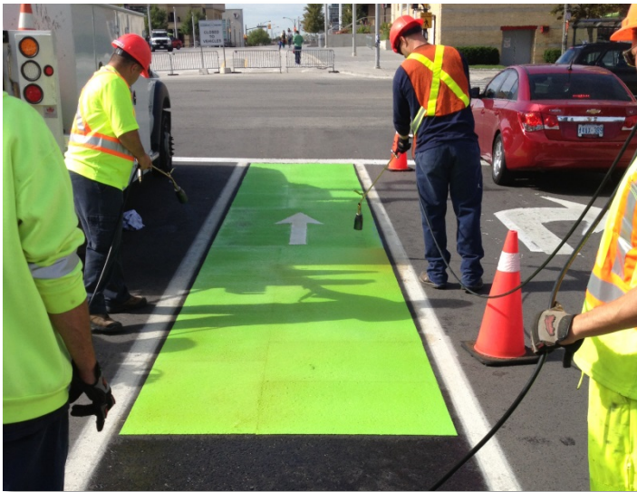
A cycling lane is painted green at Duke of York Boulevard and City Centre Drive
