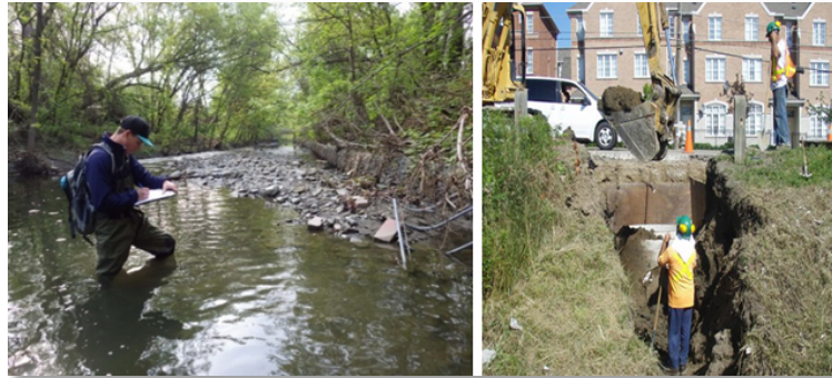
City staff evaluates a watercourse (left). Workers perform maintenance on an existing storm sewer (right)
