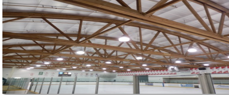
Tomken Twin Arena LED Lighting (Completed January 2014)
