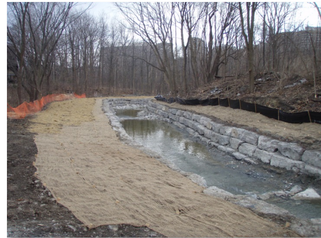
Cooksville Creek erosion control project from Burnhamthorpe Road to Mississauga Valley Boulevard
