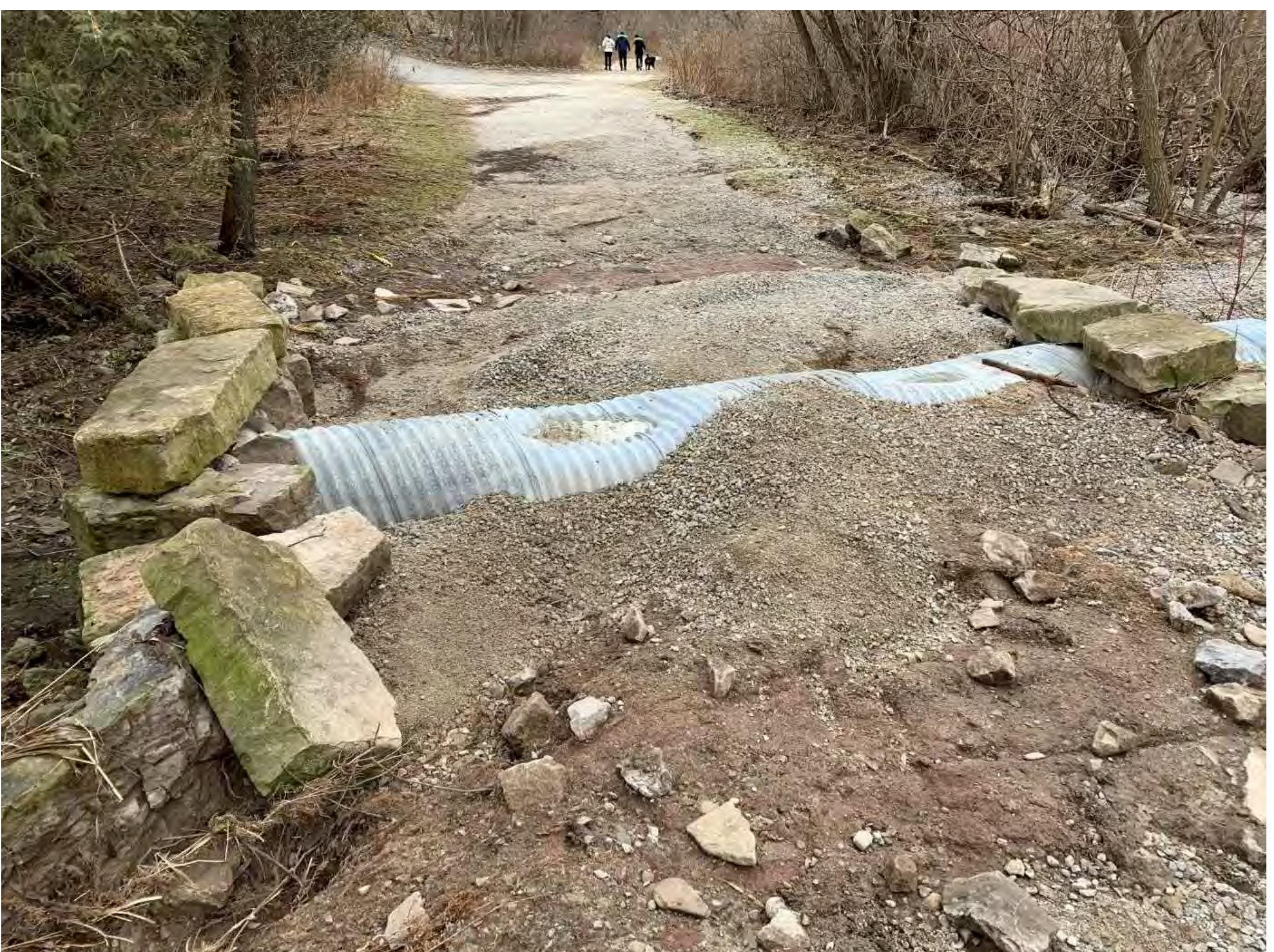
GRANULAR TRAIL WASHOUT AND EXPOSED CSP DRAINAGE PIPE
