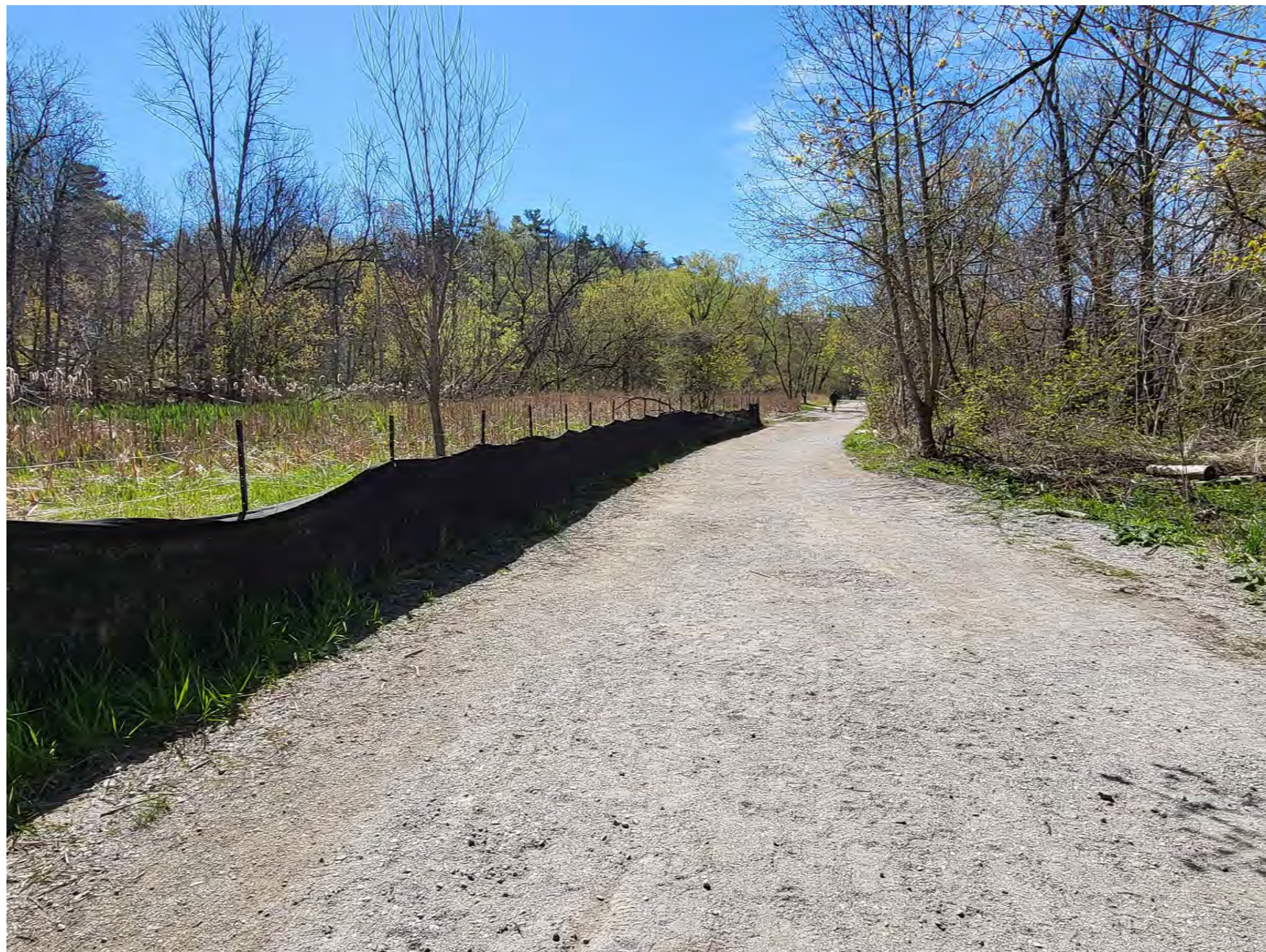
GRANULAR TRAIL PRONE TO WASHOUT ADJACENT TO TURTLE HABITAT
