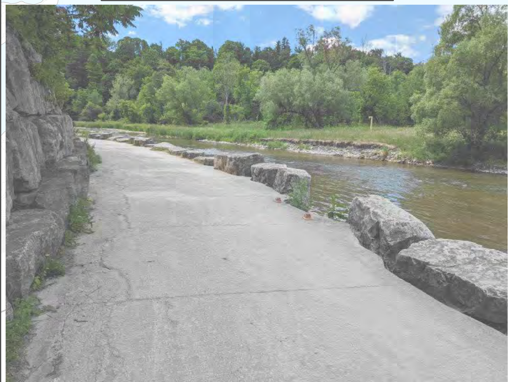
FADING ARMOURSTONE WALL AND DETERIORATED ASPHALT TRAIL
