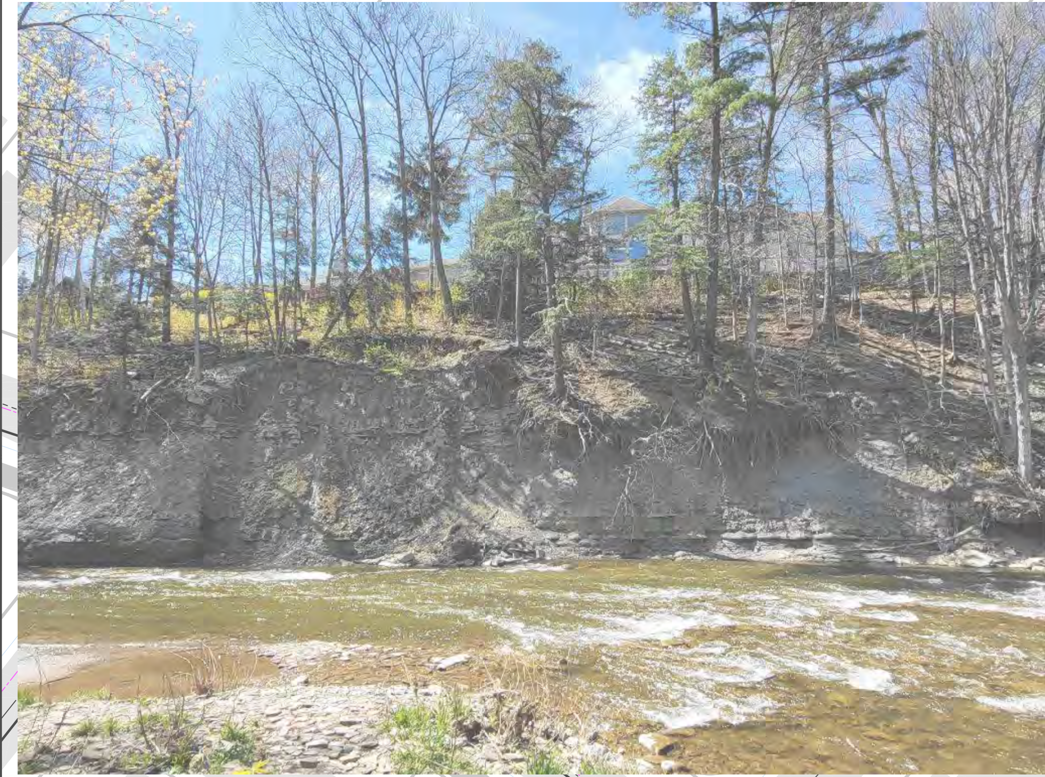
ACTIVE SLOPE EROSION
