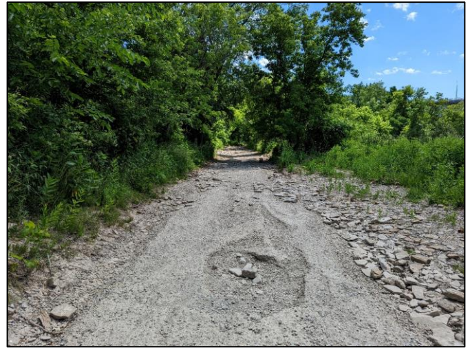
Figure 2-7: Trail Erosion Site #8 – Washout of Gravel Trail due to Frequent Flooding
