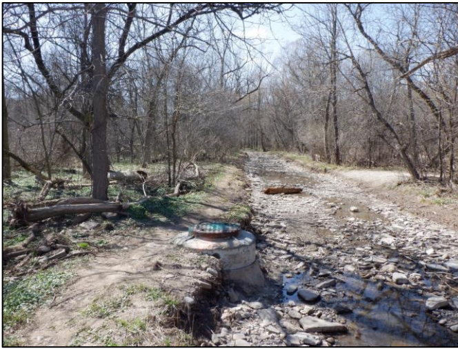
Figure 2-8: Site #8 - Degraded Sanitary Sewer Manhole Structure Along the Culham Trail
