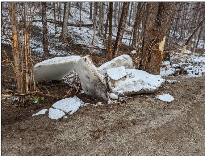
Figure 2-10: Large Chunks of Ice Debris Deposited Along the Culham Trail. Significant Tree Damage Observed.
