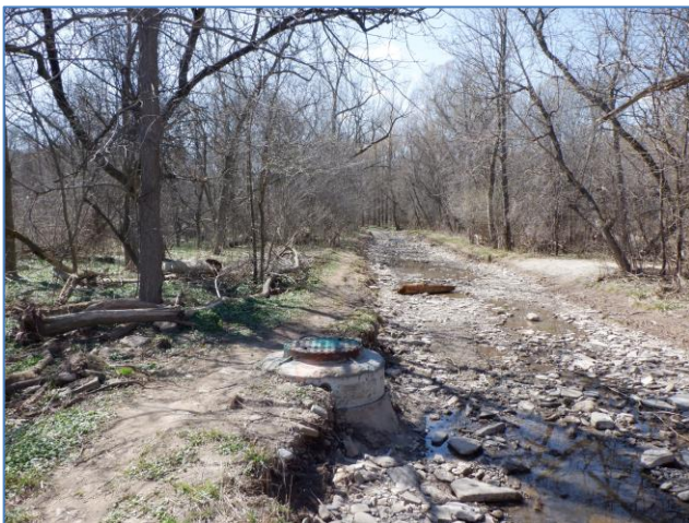
Figure 3-18: Washed Out Pedestrian Trail
