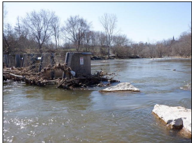
Figure 3-11: Ice Control Structure at Erindale Park
