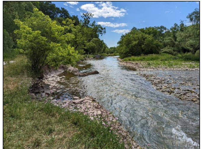
Figure 2-5: Site #3 – Failed Bank Protection Works
