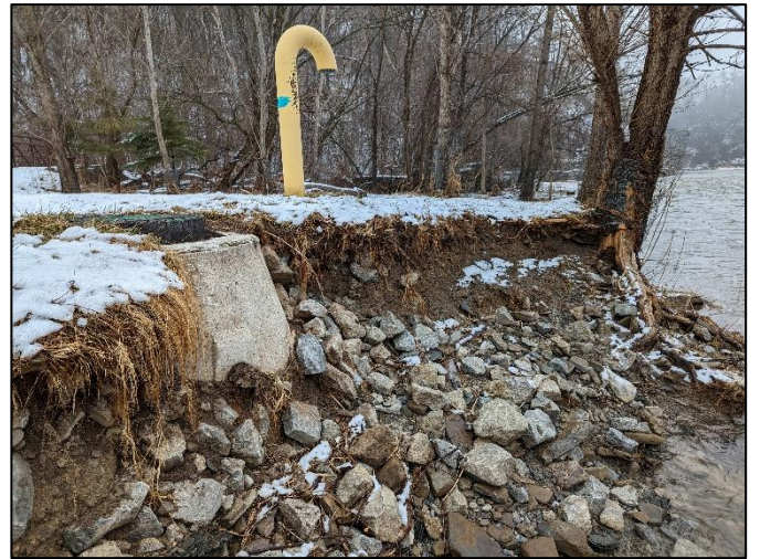
Figure 2-9: Site #7 - Exposed Sanitary Sewer Manhole Along the East Bank of the Credit River
