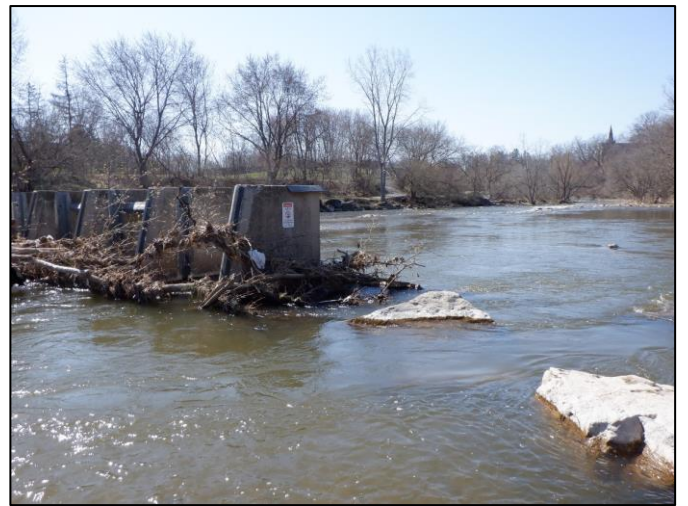
Figure 2-11: Site #1 – Outflanked Ice Control Structure Resulting from Channel Erosion Along the West Bank
