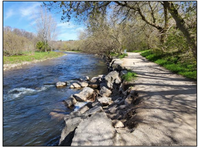
Figure 3-13: Failed Retaining Wall Adjacent to the Trail
