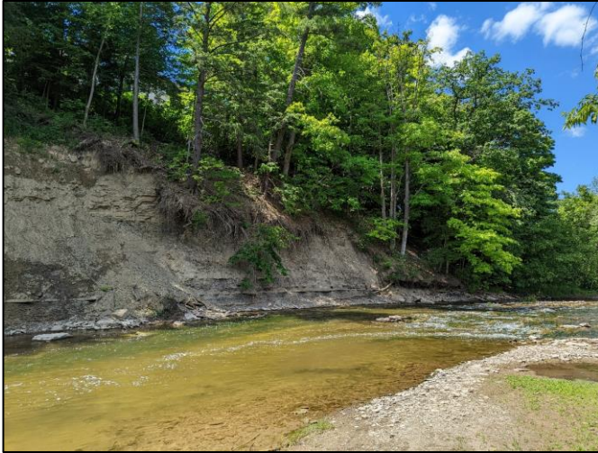
Figure 2-2: Site #5 – Slope Instability Adjacent to Private Property on Summit Court
