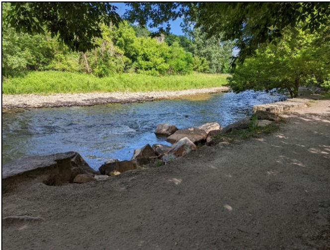
Figure 2-4: Site #2 – Failed Armourstone Retaining Wall Segment Adjoining the Culham Trail
