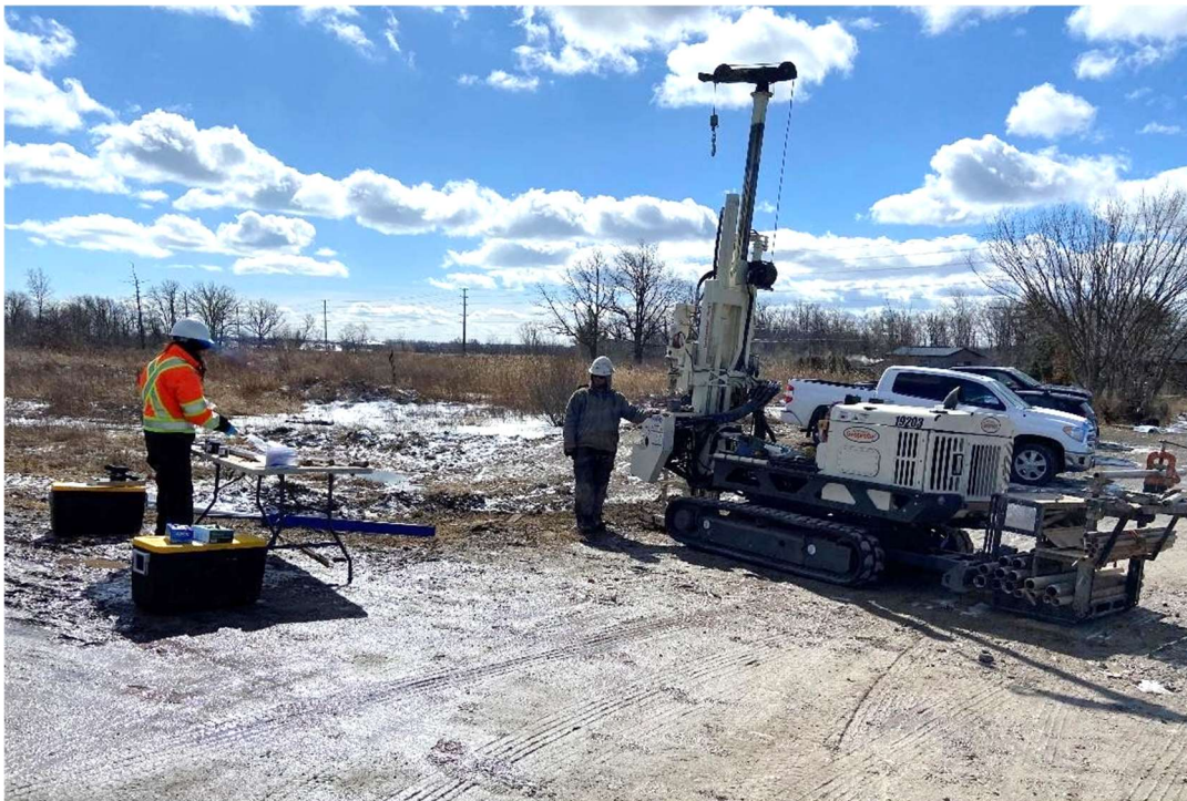
Photo 16: Looking south at Geoprobe drilling borehole BH8 near east side of the Site.
