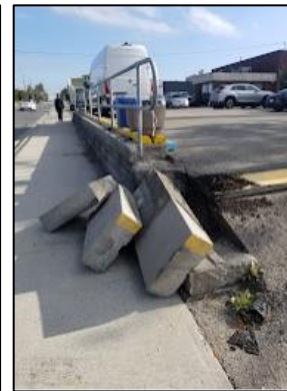
Failed Retaining Wall
