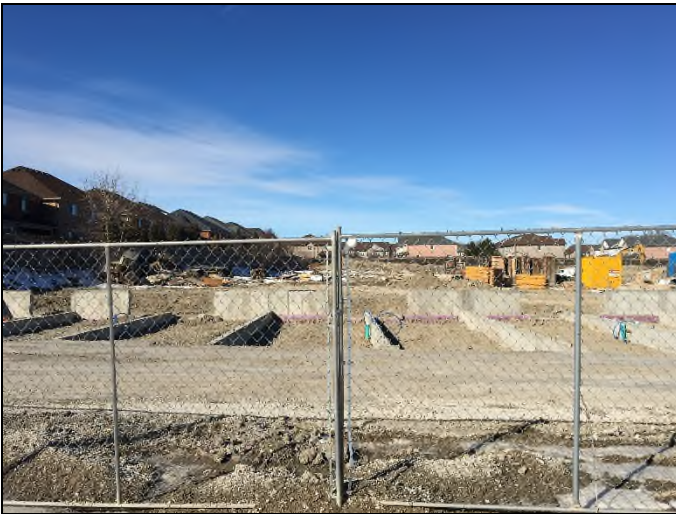
3. 80 Thomas Street – New residential development under construction located to the north of the Site.
