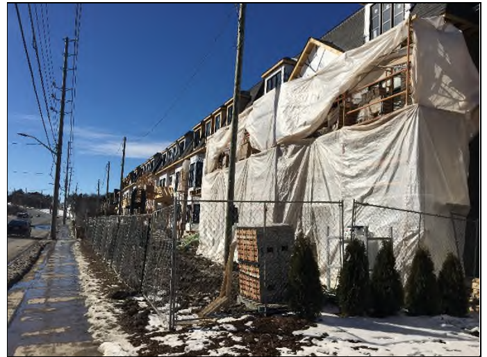
4. 80 Thomas Street – New residential houses under construction located to the east of the Site.
