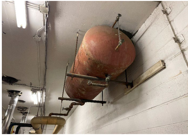
Photo #19: Aboveground storage tank suspended on the ceiling, superintendent was unsure of use, but assured it did not contain oil or fuel.
