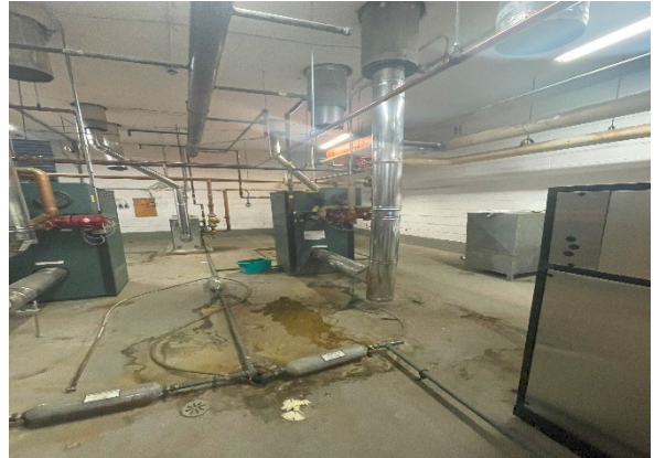
Photo #26: Boiler room located on the roof of 1850 Bloor Street.
