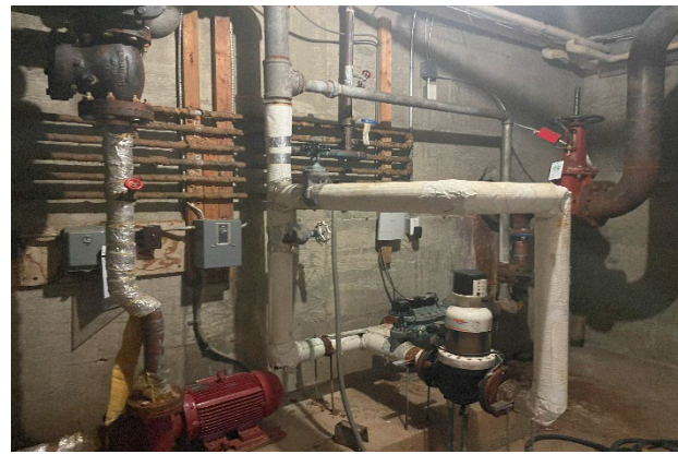
Photo #27: Pumping room located in the basement of 1850 Bloor Street.
