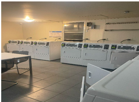
Photo #21: Laundry room located in the basement of 1840 Bloor Street.
