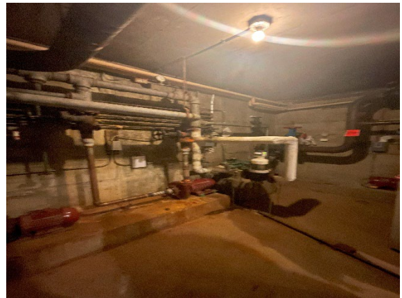
Photo #22: Pumping room located in the basement of 1840 Bloor Street.
