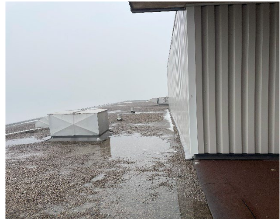
Photo #20: Ventilation fans located on roof of 1840 Bloor Street.
