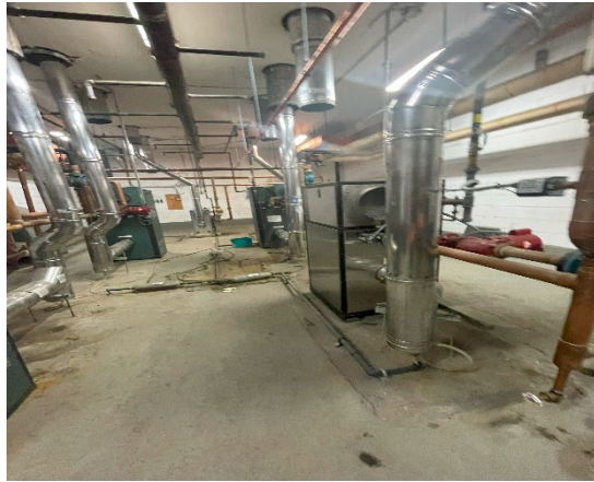
Photo #25: Boiler room located on the roof of 1850 Bloor Street.
