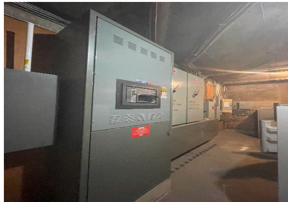
Photo #28: Electrical room located in the basement of 1850 Bloor Street.
