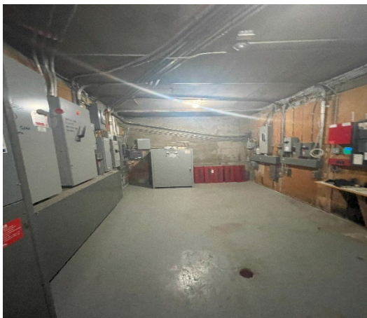
Photo #23: Electrical room located in the basement of 1840 Bloor Street.
