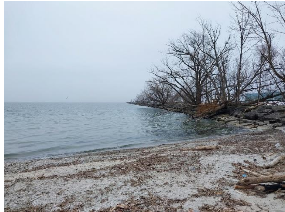
Image 54: Facing NW, edge of beach and revetment
