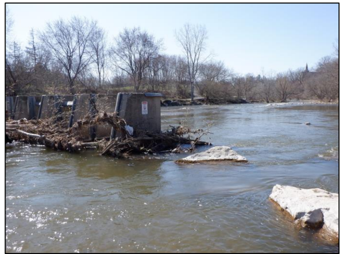
Figure 2-11: Site #1 – Outflanked Ice Control Structure Resulting from Channel Erosion Along the West Bank
