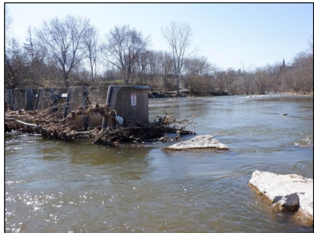
Figure 3-11: Ice Control Structure at Erindale Park
