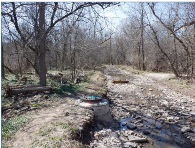
Figure 3-18: Washed Out Pedestrian Trail
