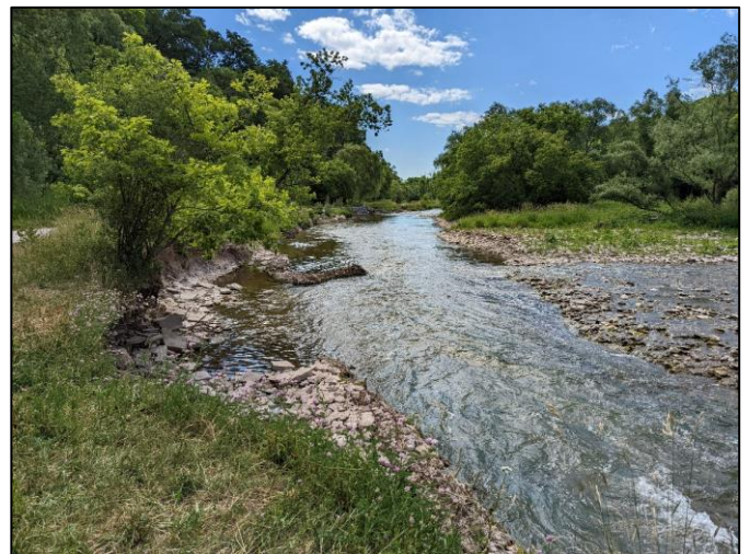
Figure 2-5: Site #3 – Failed Bank Protection Works
