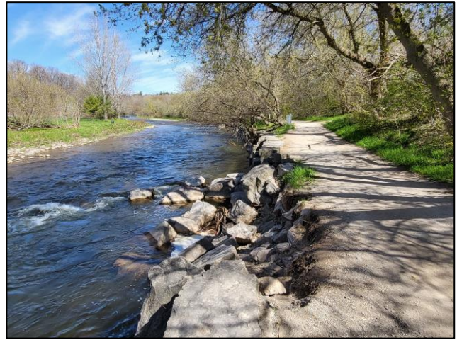
Figure 3-13: Failed Retaining Wall Adjacent to the Trail
