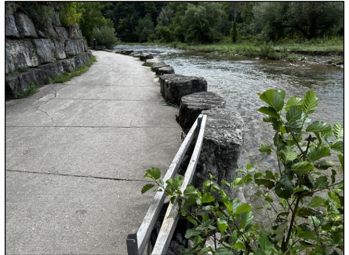
Figure 2-3: Site #4 – Failed Armourstone Retaining Wall
