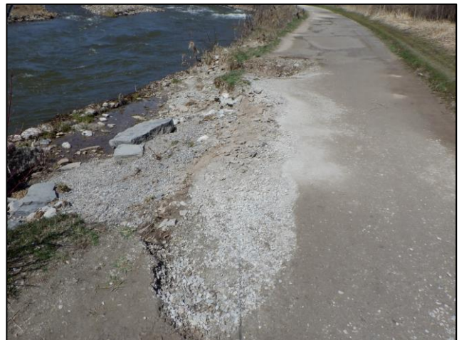
Figure 3-15: Trail Washout from Runoff and Gullying
