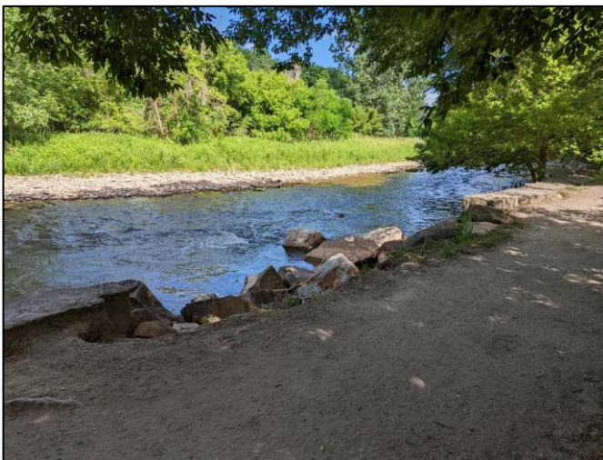
Figure 2-4: Site #2 – Failed Armourstone Retaining Wall Segment Adjoining the Culham Trail
