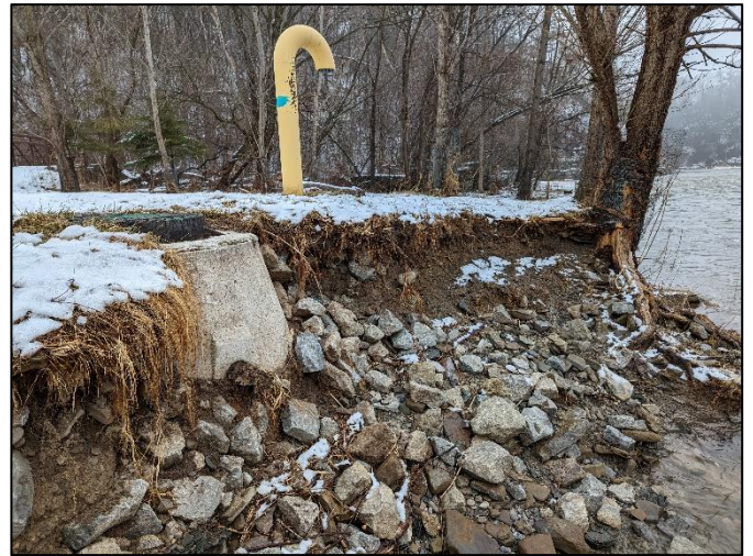
Figure 2-9: Site #7 - Exposed Sanitary Sewer Manhole Along the East Bank of the Credit River
