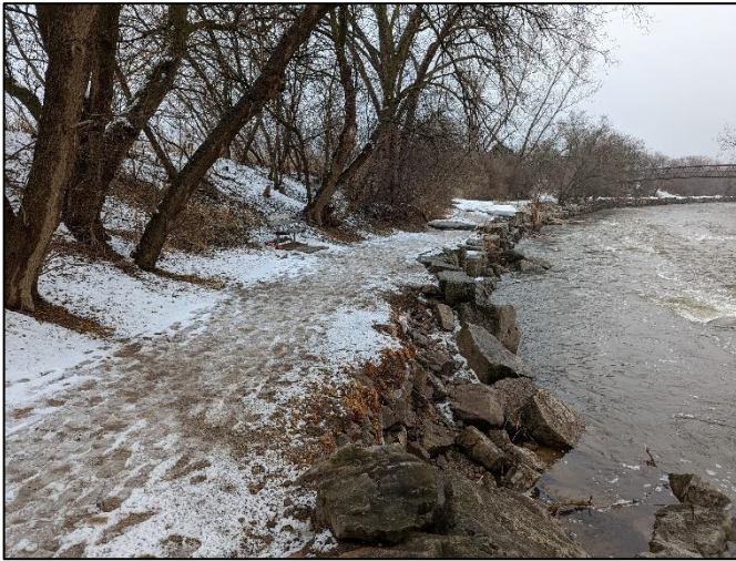
Figure 2-6: Site #6 – Failed Armourstone Retaining Wall Segment Adjoining the Culham Trail
