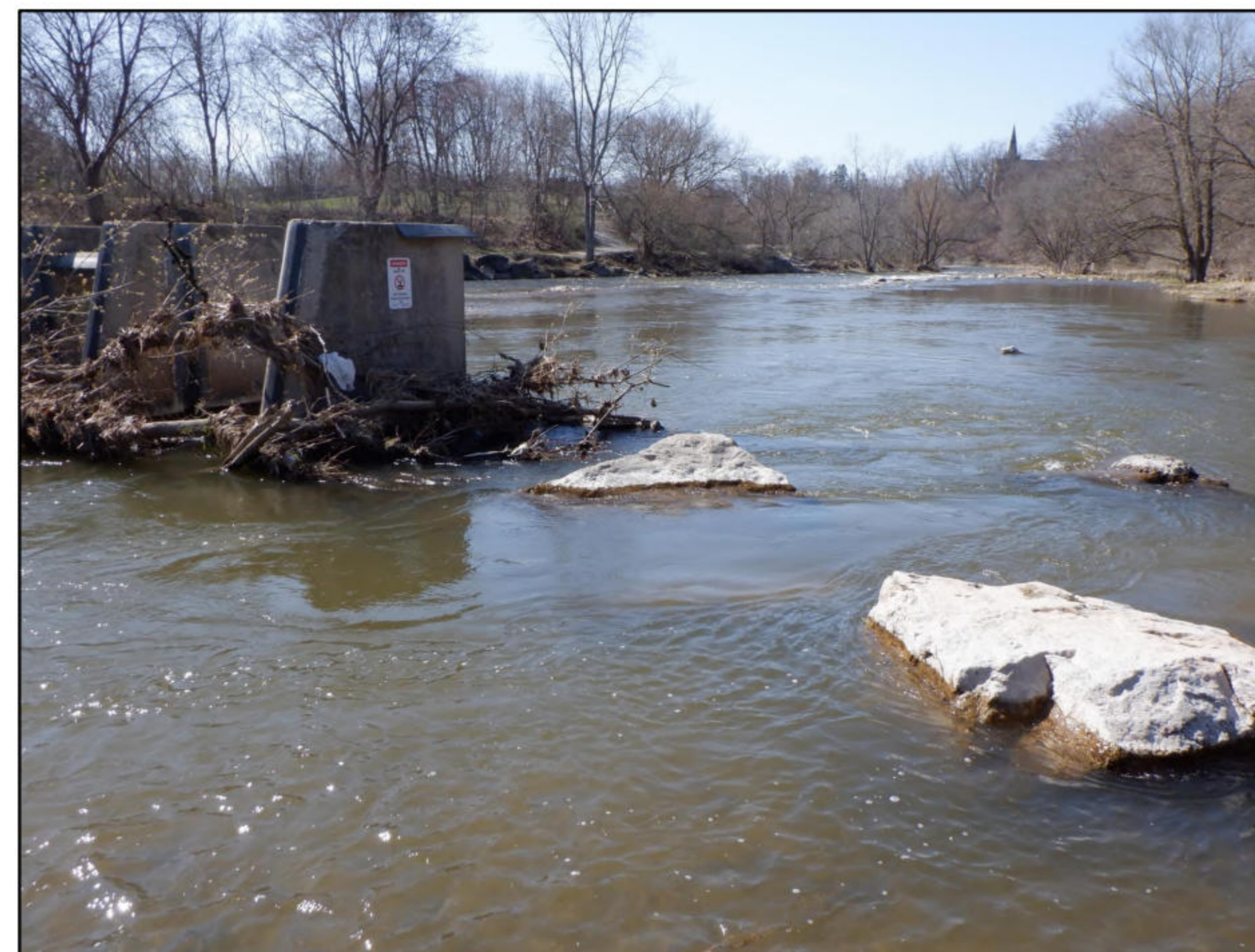
By-Passed Ice Control Structure
