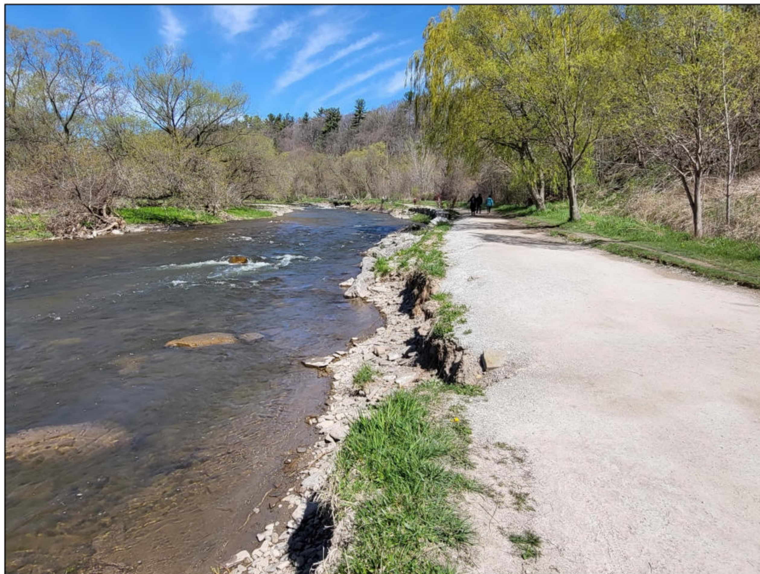
Bank Erosion Along Culham Trail
