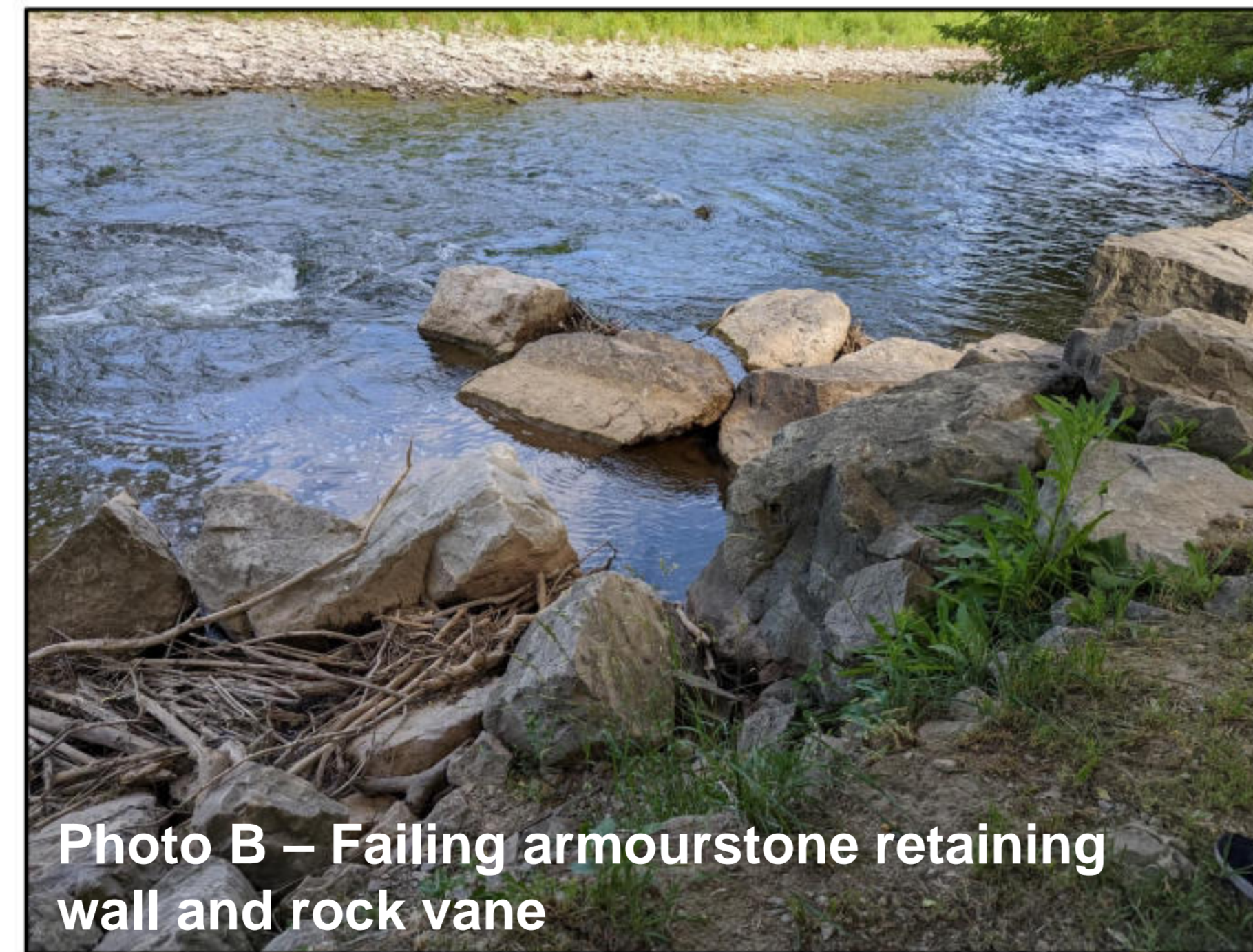
Photo A – Failing armourstone retaining wall adjacent to trail
