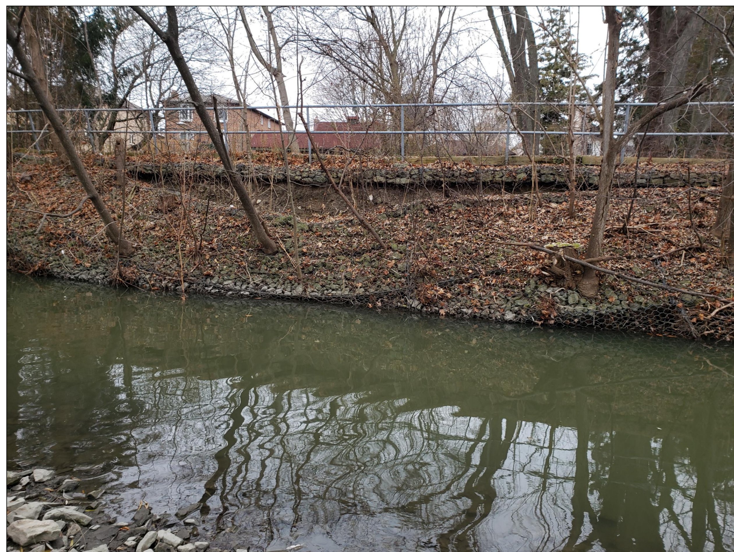
Deteriorated Gabion Baskets Throughout Study Area
