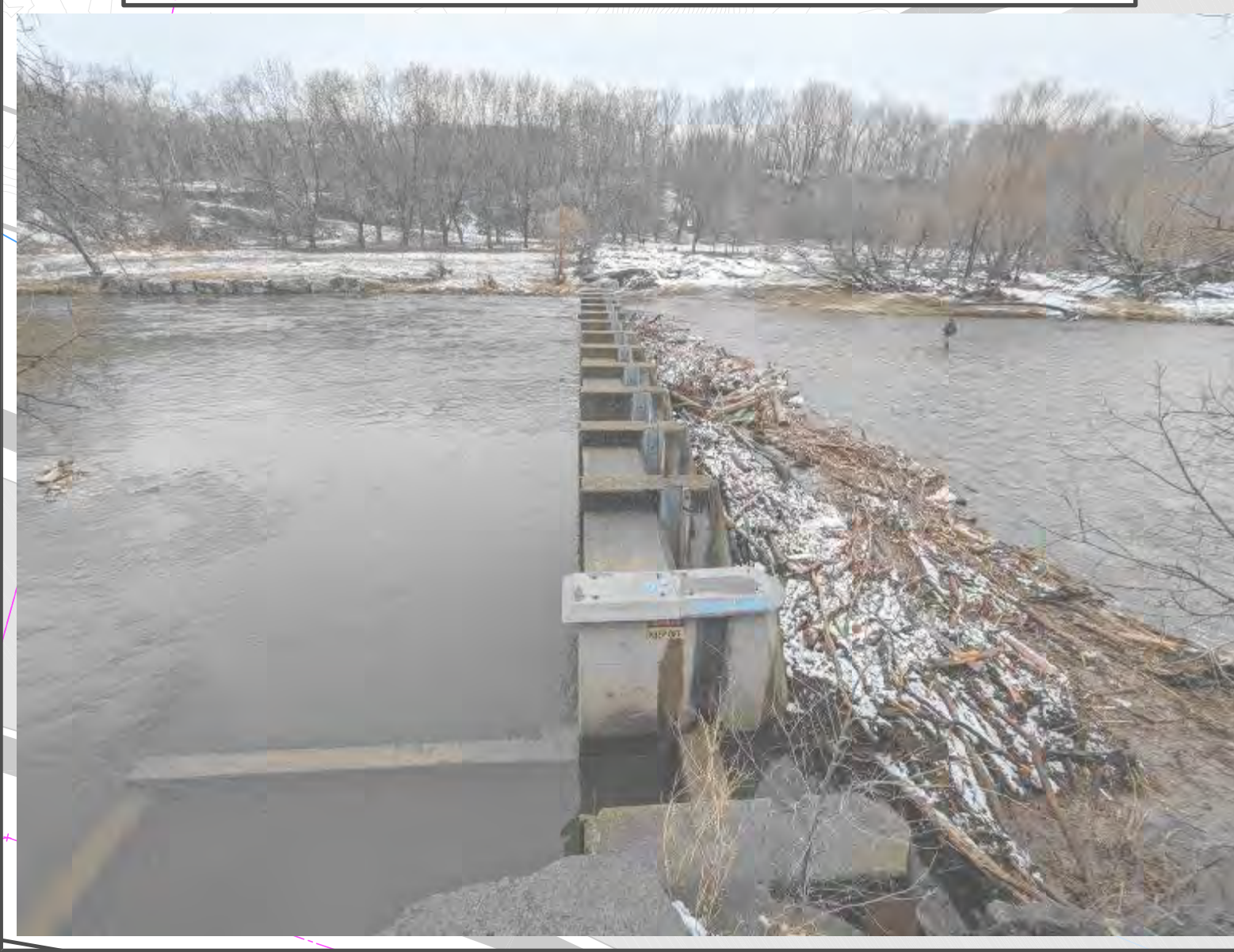
FAILING ARMOURSTONE WALL, BANK EROSION AND DEBRIS ACCUMULATION
