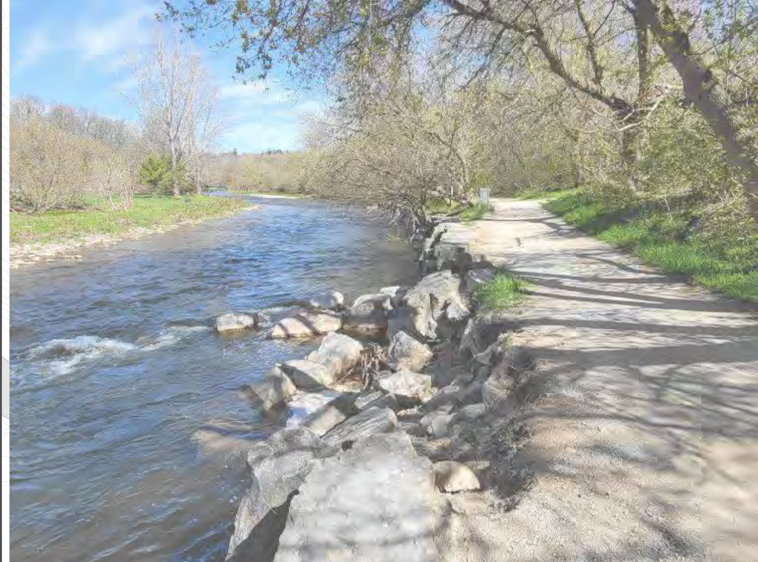
FAILING ARMOURSTONE WALL AND STONE WEIRS
