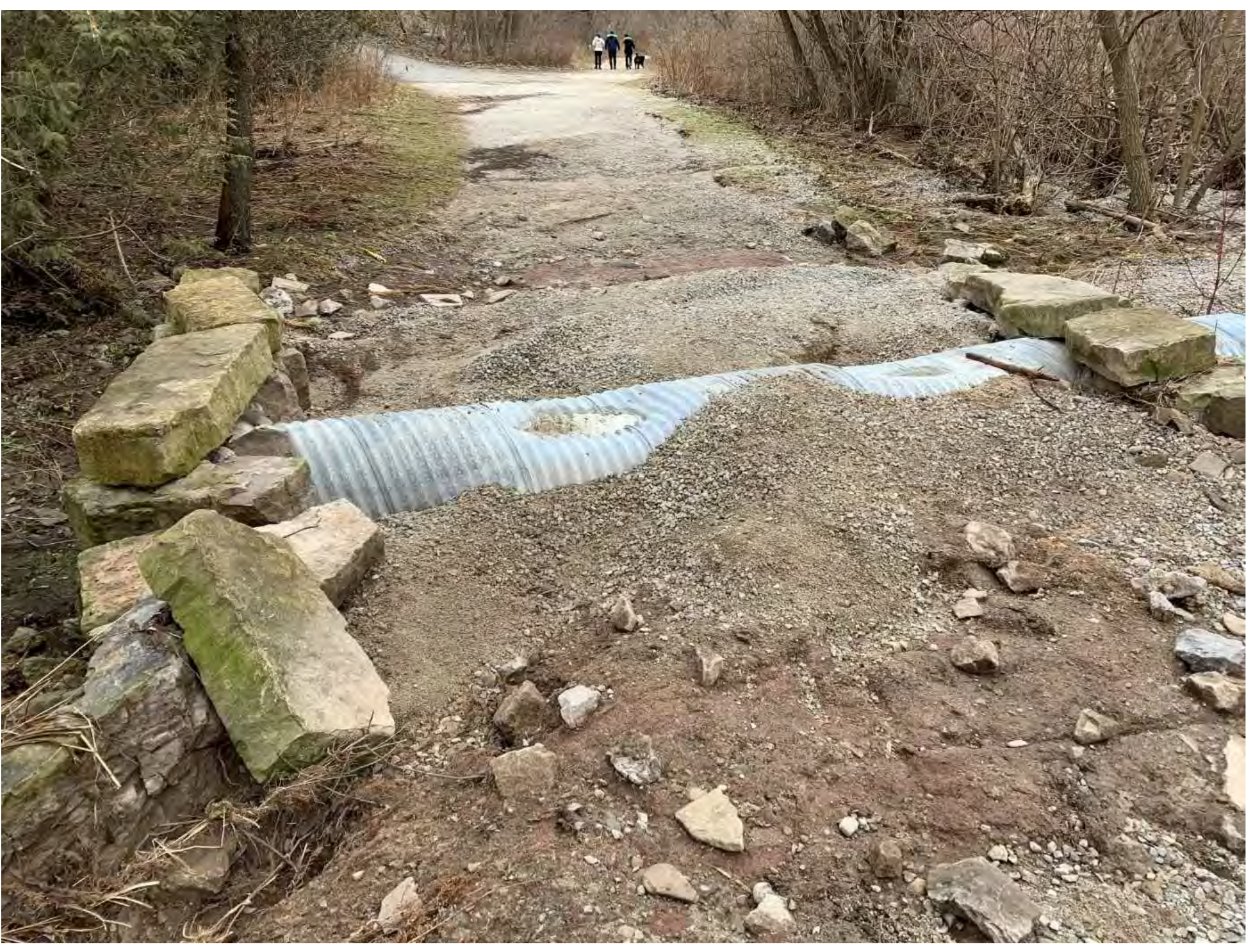
GRANULAR TRAIL WASHOUT AND EXPOSED CSP DRAINAGE PIPE
