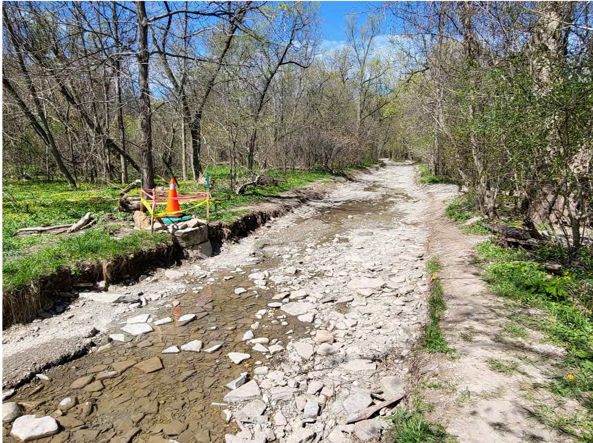
GRANULAR TRAIL WASHOUT AND EXPOSED SANITARY MANHOLE
