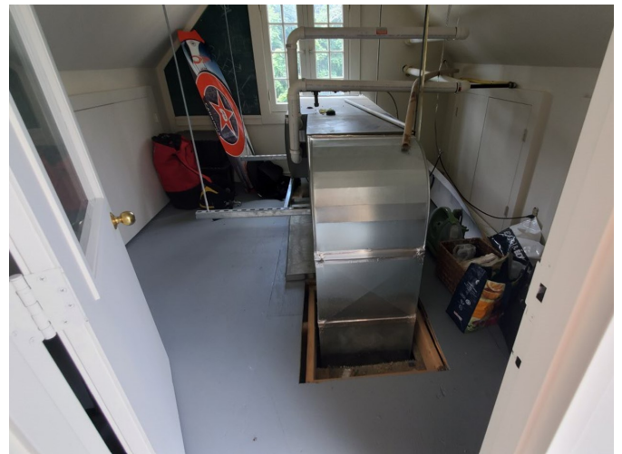
Photo 10: View of the HVAC system, located on the third floor of Site Building B.
