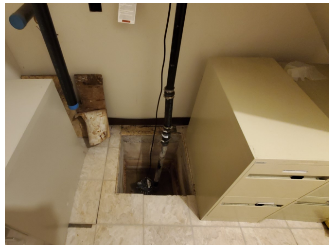
Photo 18: View of the sump pump, within the basement of Building D.
