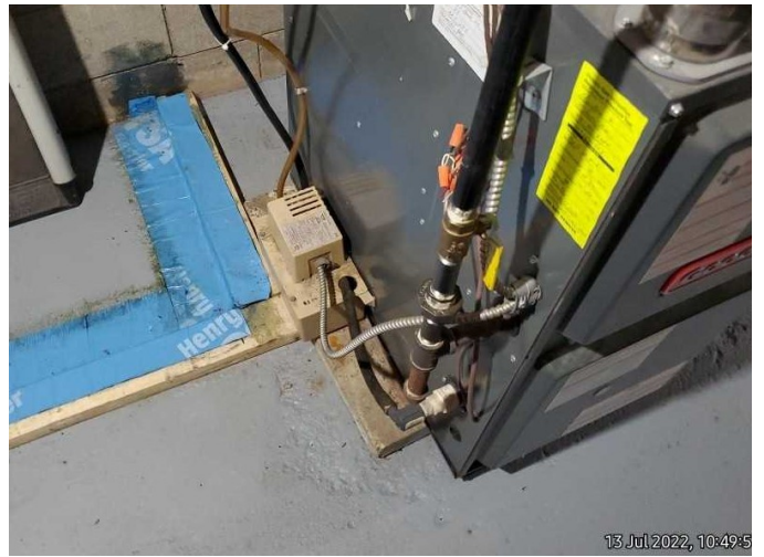
Photo 14: View of the natural gas furnace, located within the basement of the Site Building C.
