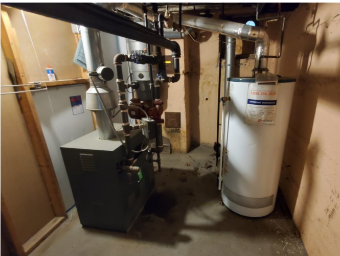
Photo 9: View of natural gas furnace and hot water tank, located in the basement of Site Building B.
