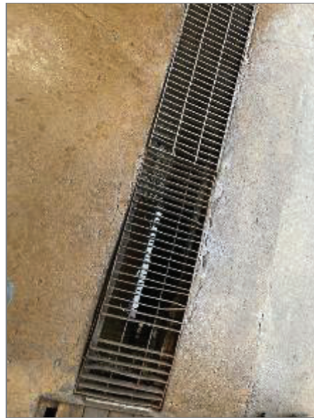
Photo 12 – OWS trench in south portion of Site Building C.
