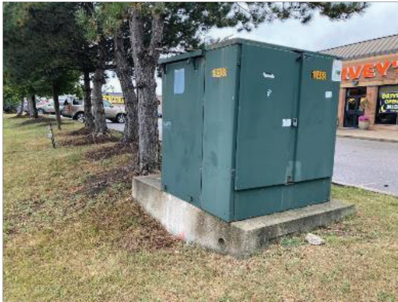
Photo 15 – Transformer in east corner of Phase One Property.
