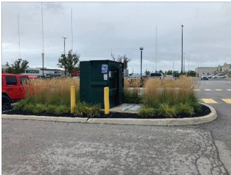
Photo 20 – One of two transformers at 970 Southdown Road, 90 m southeast of the Phase One Property.
