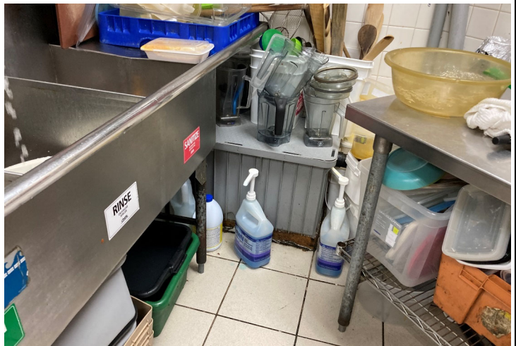
Photo 16: General grease interceptor observed in restaurant tenants.
