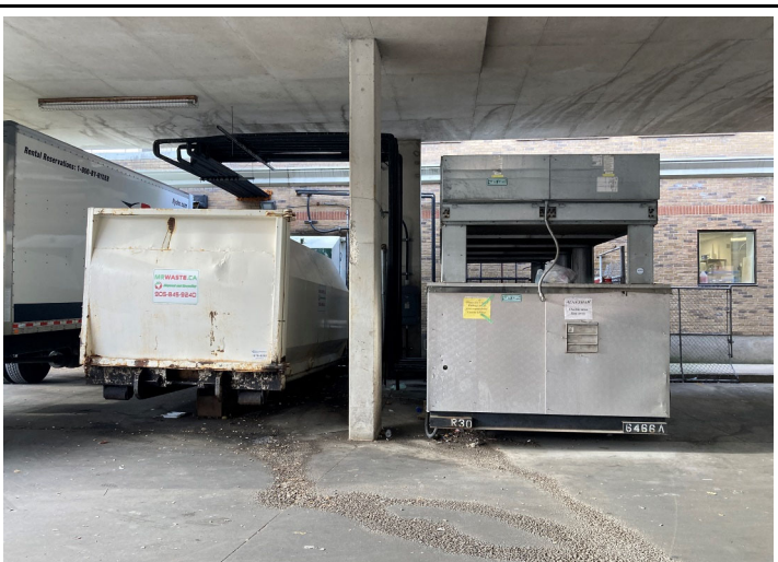
Photo 8: Refrigerant compressor and garbage compactor for Al-Najmah Fine Foods supermarket, facing southwest.
