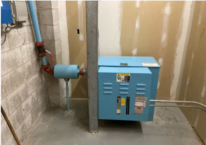
Photo 13: Elevator maintenance room. No staining observed or reported.
