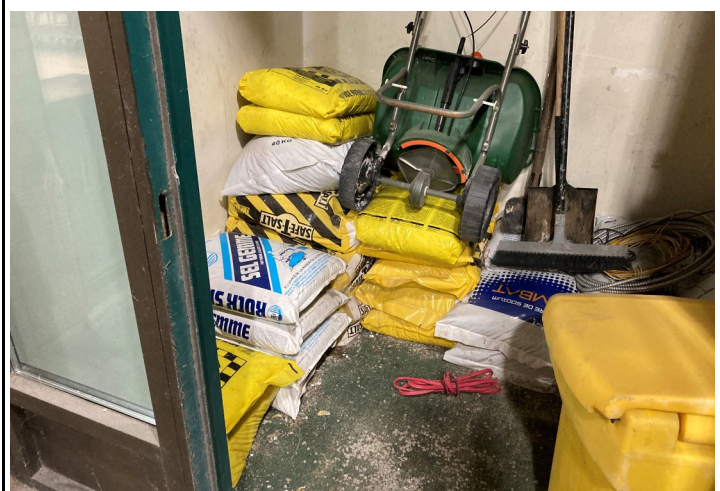
Photo 11: Bulk storage of salt for de-icing measures located in sprinkler room.
