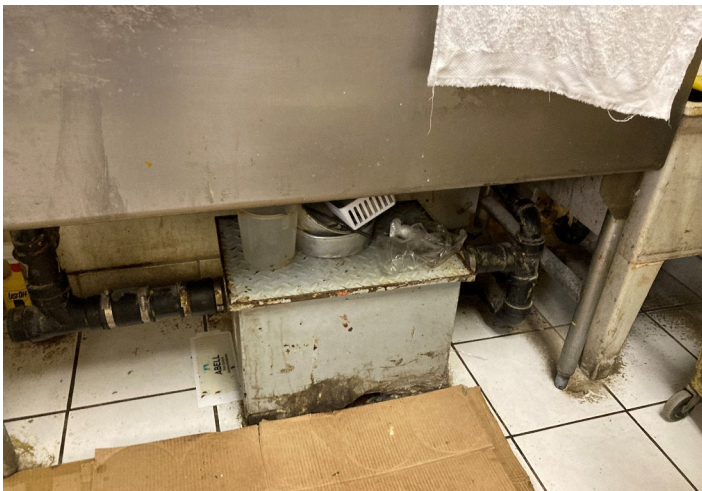
Photo 15: General grease interceptor observed in restaurant tenants.
