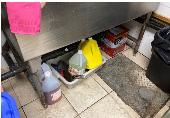
Photo 17: General grease interceptor observed in restaurant tenants.
