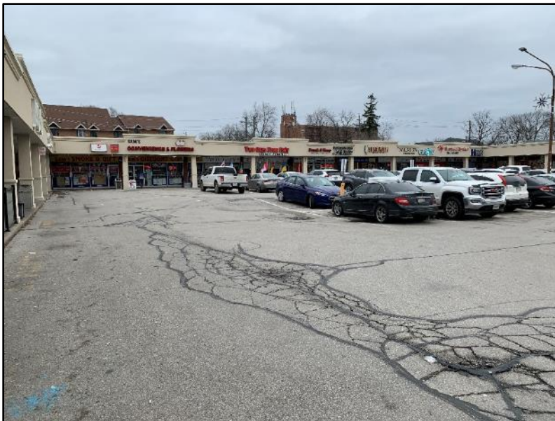
Image 2: View of the main 'L'-shaped commercial building, with a paved asphalt parking lot.
