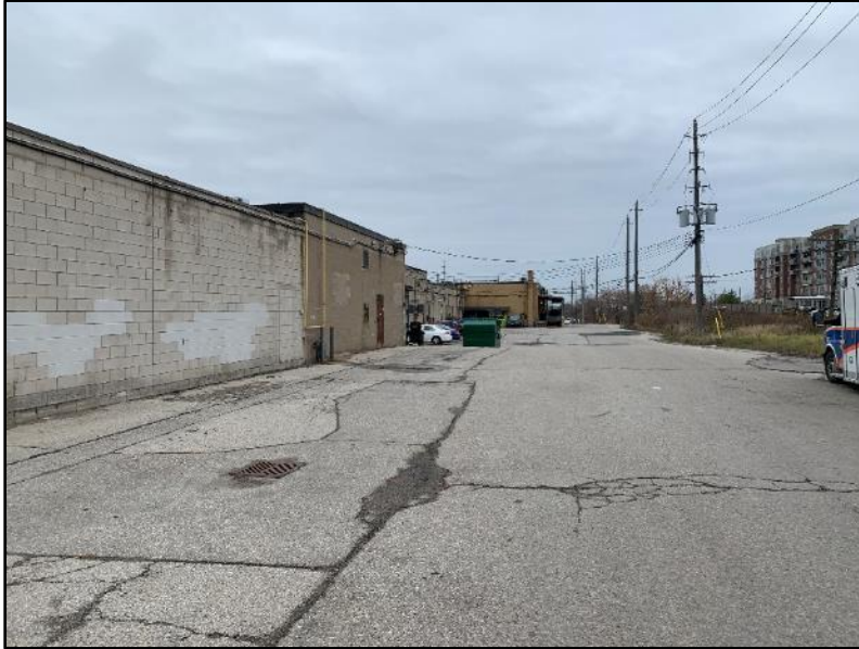
Image 3: Rear view of the main 'L'-shaped commercial building with paved asphalt access laneway and storm water catch basin.
