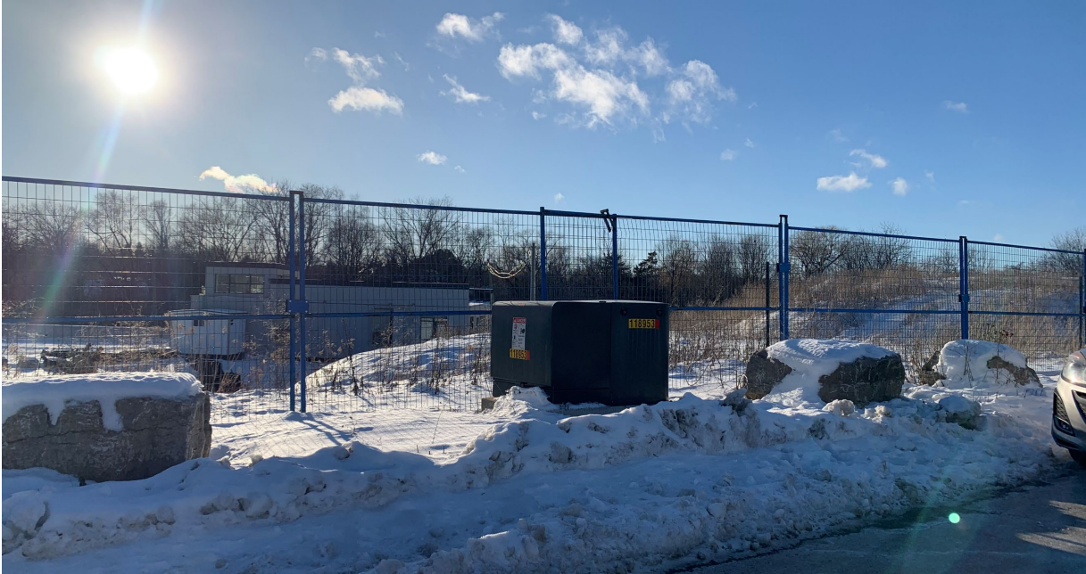
Photo 15 View of transformer located on southeastern portion of Site, facing west
