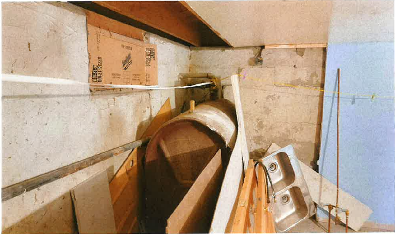
View of fuel oil AST located in the basement of the house in the northern portion at the subject site
