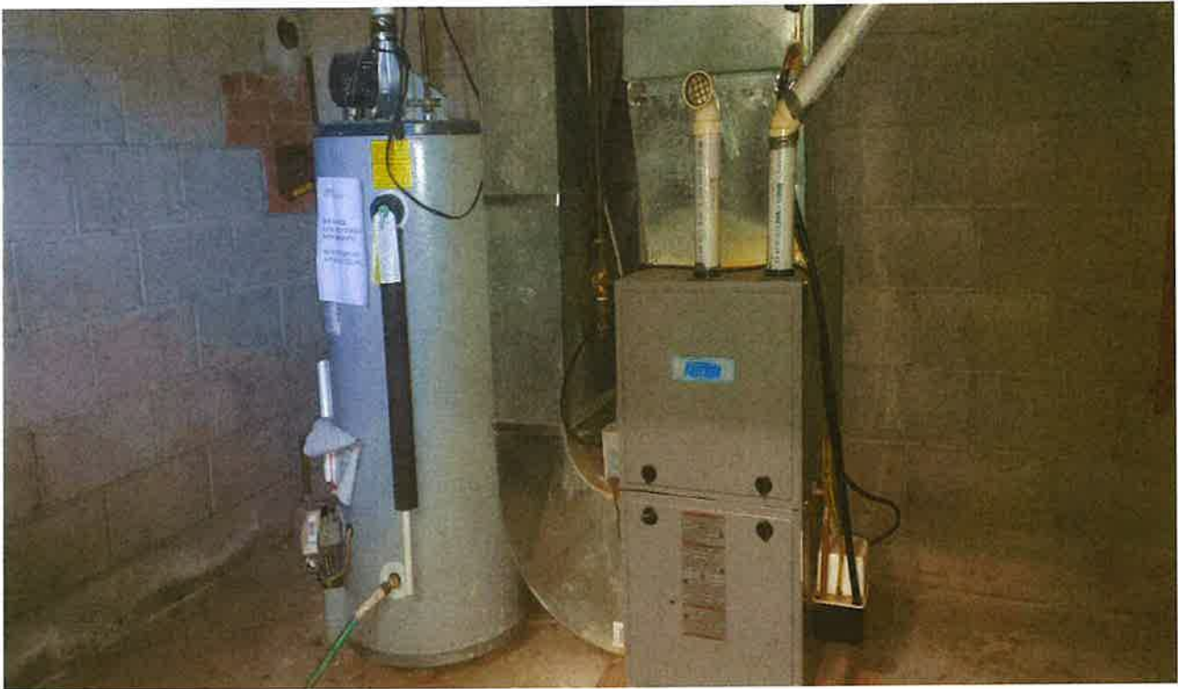
View of water heater and furnace in the basement of the house (looking northwest)
