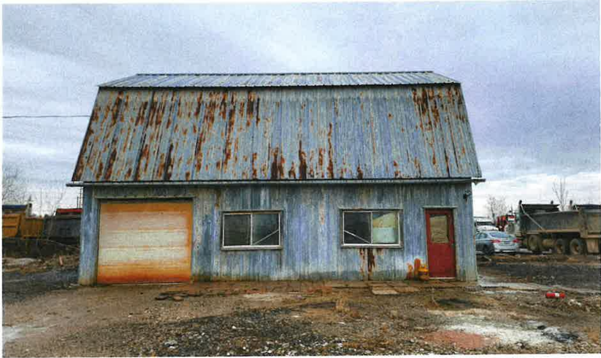
View of a shed located in the north-eastern portion of the subject site (looking northeast)
