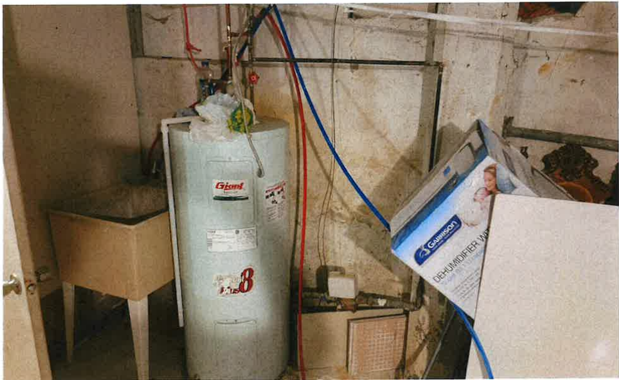
View of water heater in the basement of the house at the subject site
