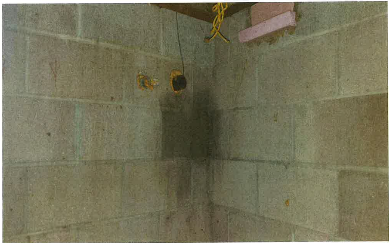
View of filler pipe in the basement of the house (looking northwest)
