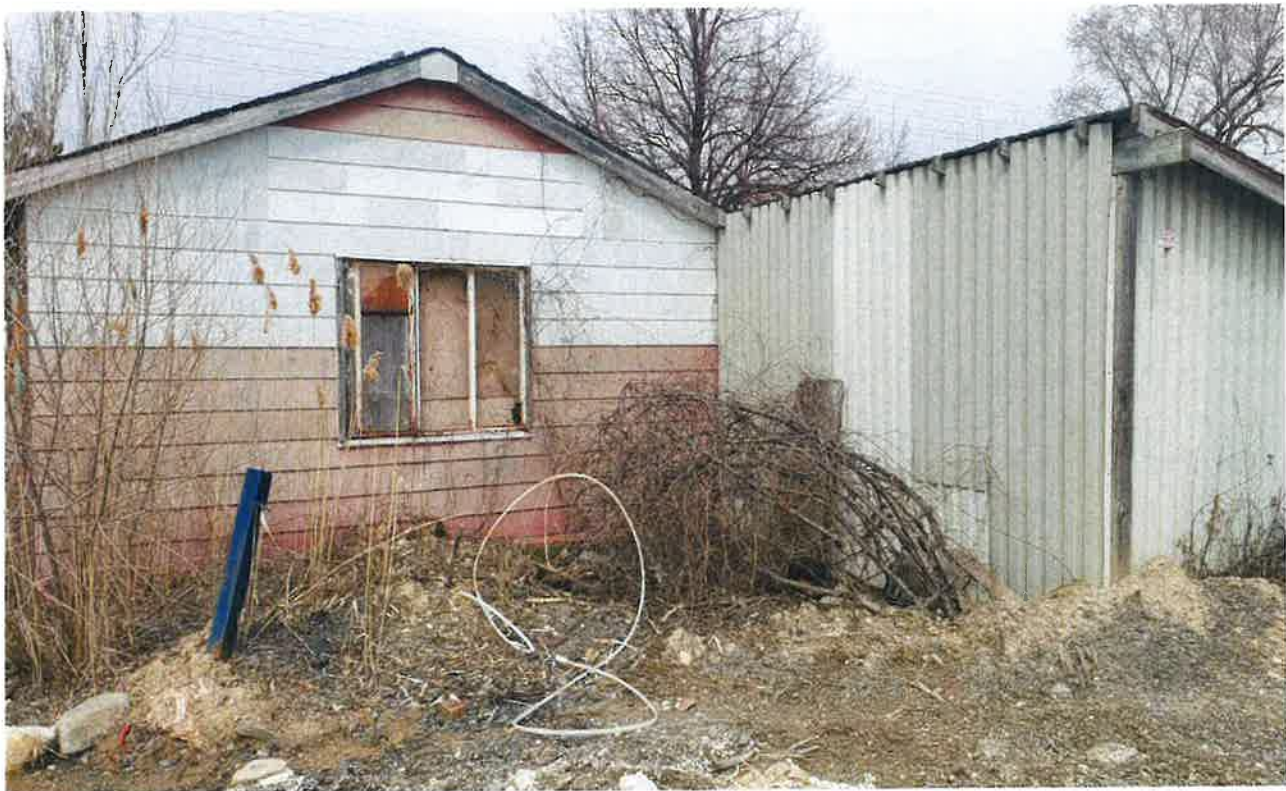
View of the detached car garage in the western portion of the subject site (looking north)
