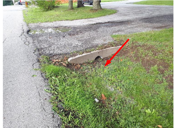
Photo 10: View of a portion of the drainage ditch (see arrow) located on the south portion of the Subject Property.
