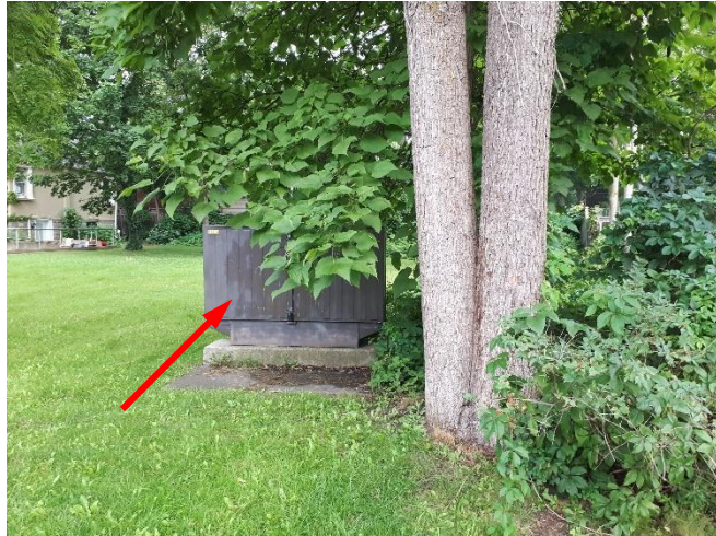
Photo 9: View of the concrete pad mounted transformer (see arrow) located on the southeast portion of the Subject Property.
