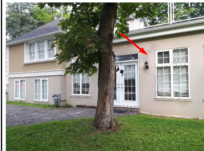
Photo 3: View of a portion of the south elevation (see arrow) of the Subject Building, looking northwest.
