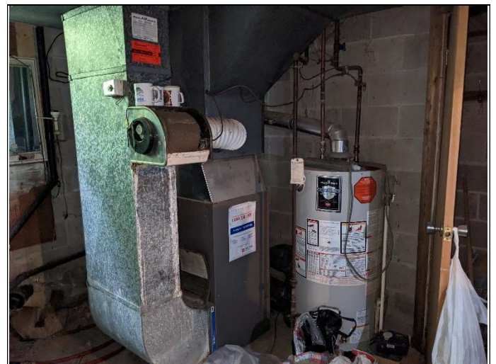
6. View of the boiler room located in the basement of the on-site dwelling.
