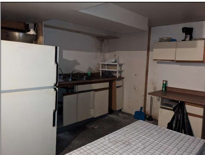
5. View of the kitchen in the basement of the on-site dwelling and signs of water stains/mould.
