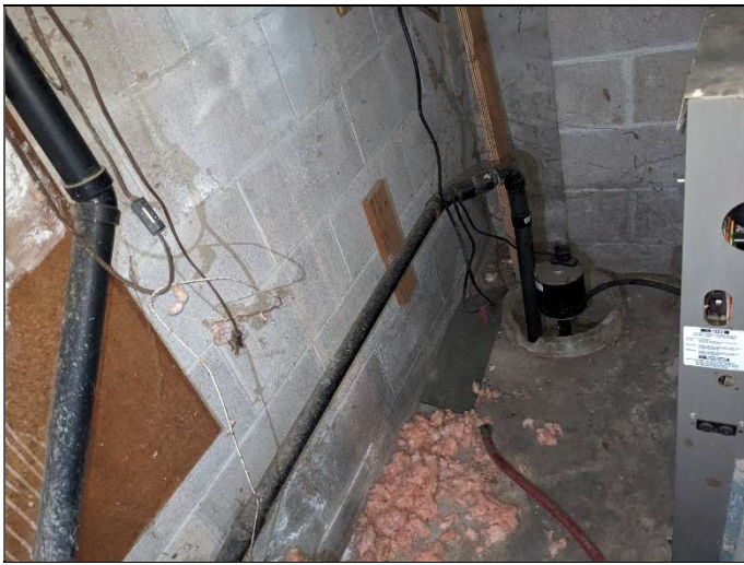
7. View of sump pump behind the HVAC system in the basement of the on-site dwelling.
