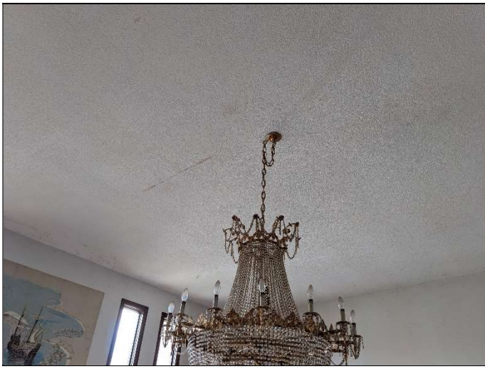
13. View of the water stains on the ceiling located in the main area of the on-site dwelling.
