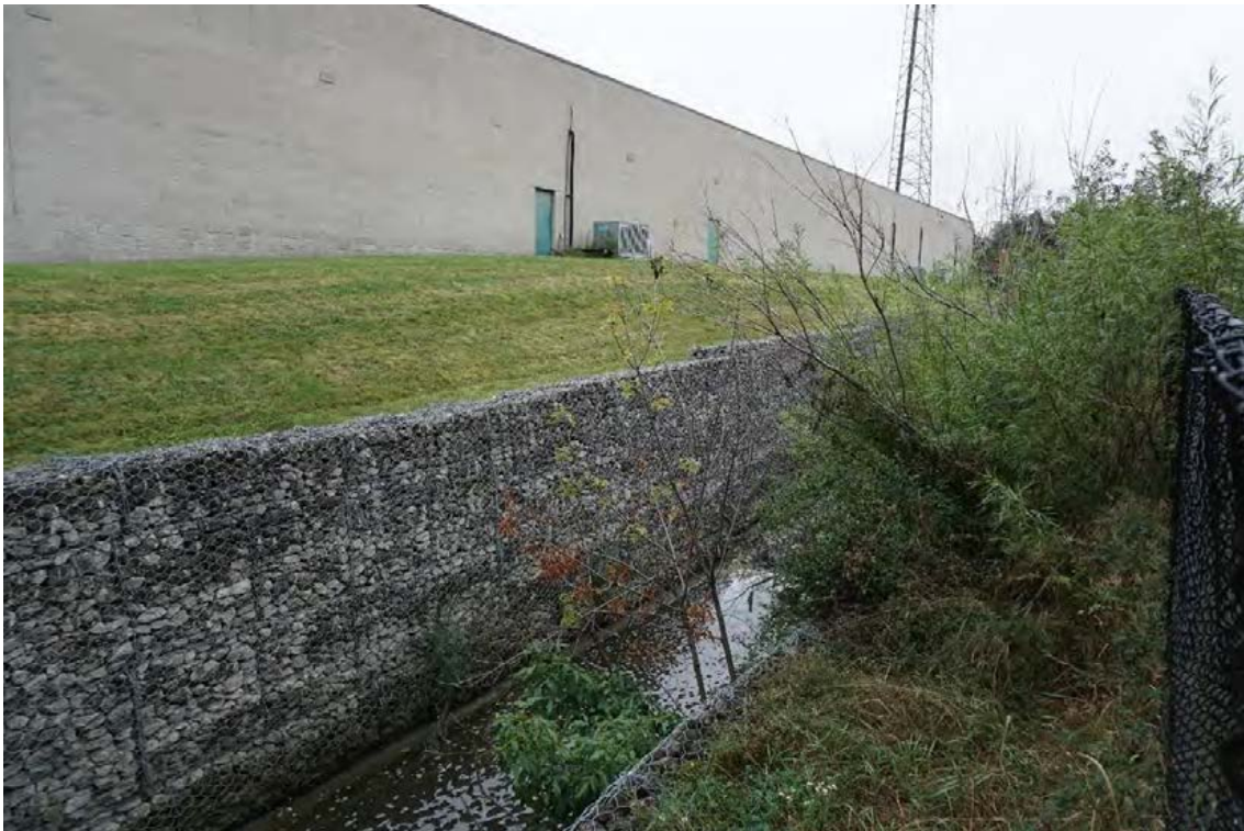
Photograph 2: View of the channelized segment of Wolfedale Creek located in Study Area 1 (AECOM 2023)
