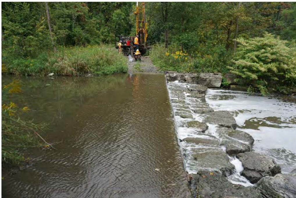
Photograph 11: View of Wolfedale Creek located in Study Area 2, the armour stone/concrete retaining wall and the surrounding low-lying riparian area, looking east (AECOM 2023)
