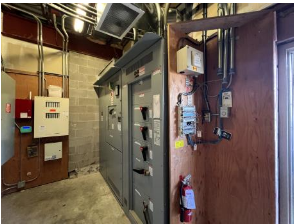
Photo 15: View of the interior of the electrical room for Site Building A. Photograph taken facing southwest
