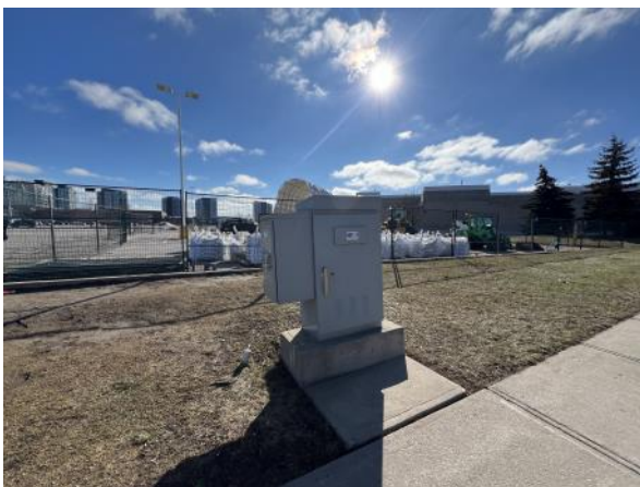
Photo 33: View of the traffic control panel along northern boundary of Phase One Property. Photograph taken facing south.
