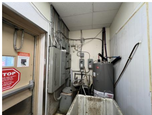
Photo 24: View of the Electrical Panels, hotwater tank inside Pizza Pizza. Photograph taken facing northwest.
