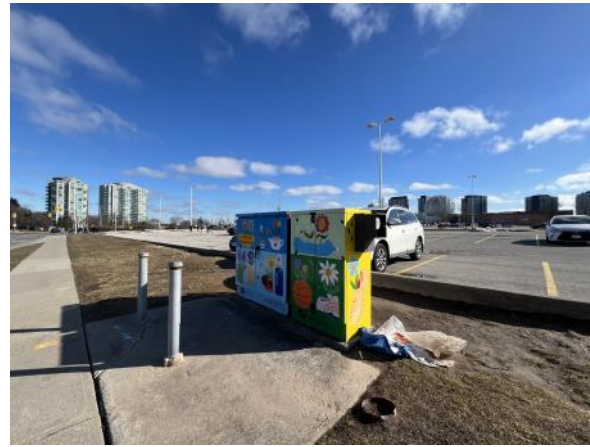
Photo 32: View of the transformers along the north boundary of Phase One Property. Photograph taken facing southeast
