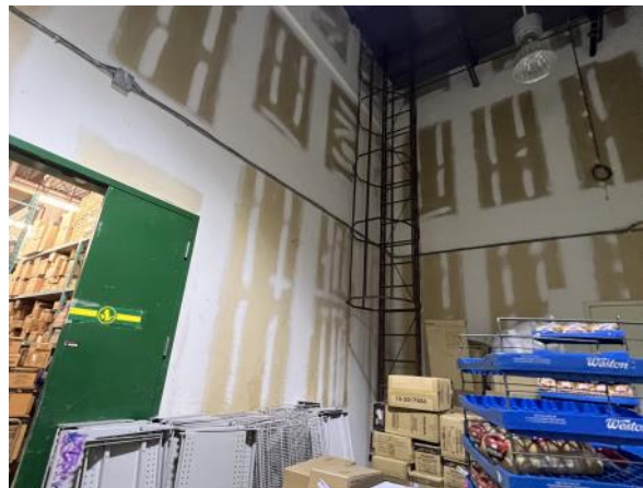
Photo 10: View of the stairway providing roof access and backdoor to Dollarama from loading bay area/ room of Site Building A. Photograph taken facing south.
