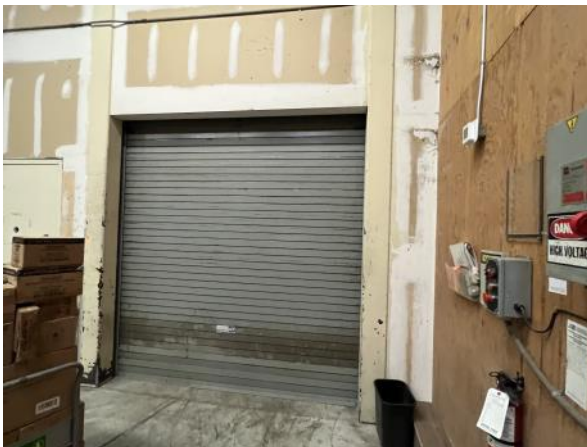
Photo 9: View of the electric garage door in the loading bay area/ room of Site Building A. Photograph taken facing southwest.
