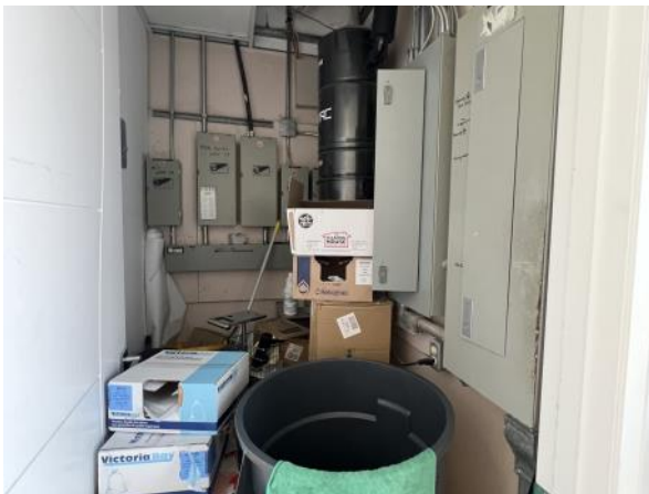
Photo 27: View of the electrical panels inside the walk-in medical clinic. Photograph taken facing north.
