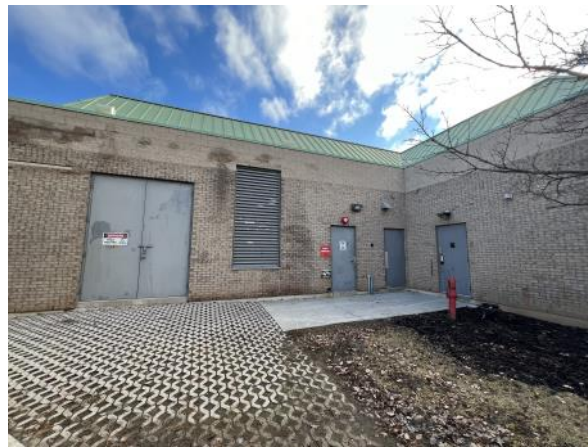
Photo 16: View of the doorway leading to electrical rooms / sprinkler system access to Site Building B. Photograph taken facing southeast.
