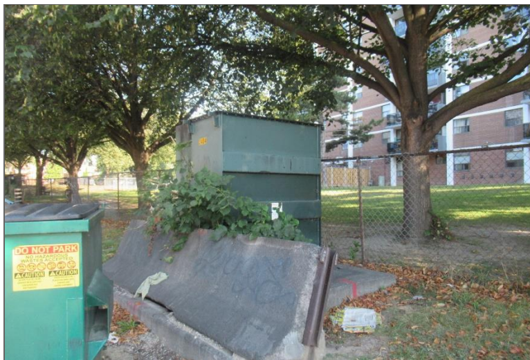
Photo 10 – Pad-mounted transformer located along the northcentral side of 3405-3445 Fieldgate Drive.
