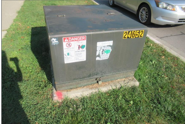
Photo 9 – Pad-mounted transformer located along the northeast side of 1835 Bloor Street.
