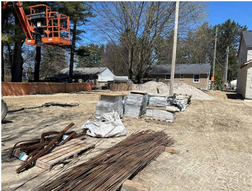
Image 6: View north across area of grading in the south of the subject property from the south corner.
