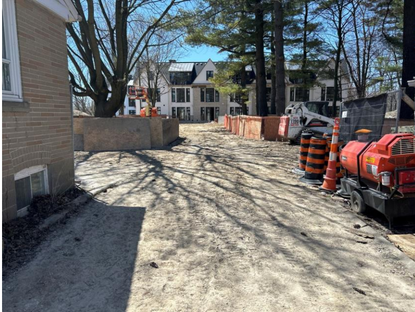
Image 5: View west between the two houses. Note the grading that extends past the southwest limit of the subject property.
