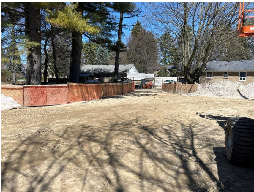
Image 2: View of extensive grading through the backyard areas of the subject property, looking north from the south corner.
