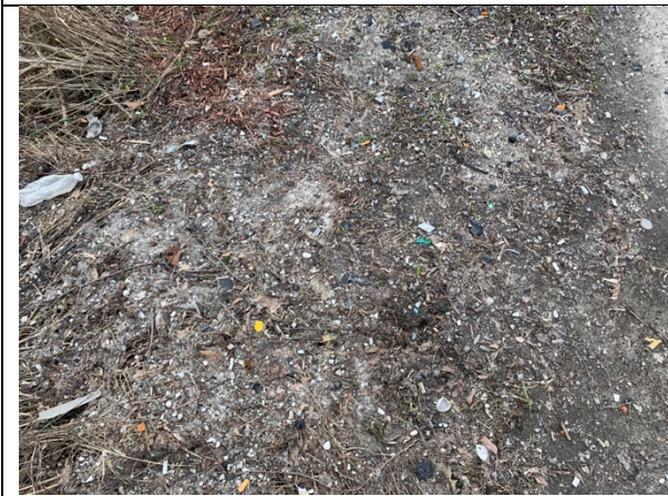
IMAGE 3 GRAVEL AND ASPHALT AT TOP OF SLOPE
